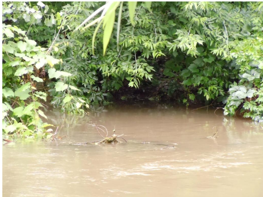
Same storm sewer outlet on June 26, 2013, 9:55:08 AM. Stormwater is actively flowing out of the pipe into Wingra Creek due to recent heavy rain. The top of the pipe is completely underwater in this image. During periods of normal summer water levels at least half of this three foot diameter pipe is above water.
